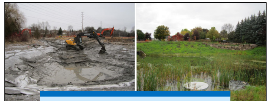
Construction at retrofit #1, George Richardson in Newmarket (left); Post construction at retrofit #2, Colony Trial in East Gwillimbury (right).
